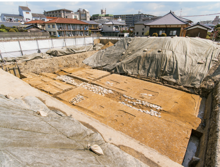
西大寺旧境内（薬師堂西方）の発掘調査 Excavation in the former precinct of Saidaiji temple (west of Yakushidō)
