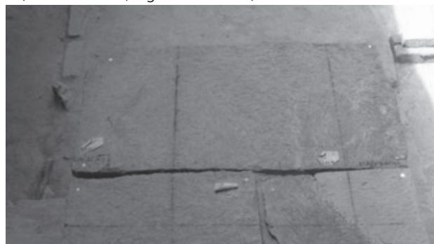
Fig. 42: South stairways of the Central Sanctuary view of the west top surface after restoration
