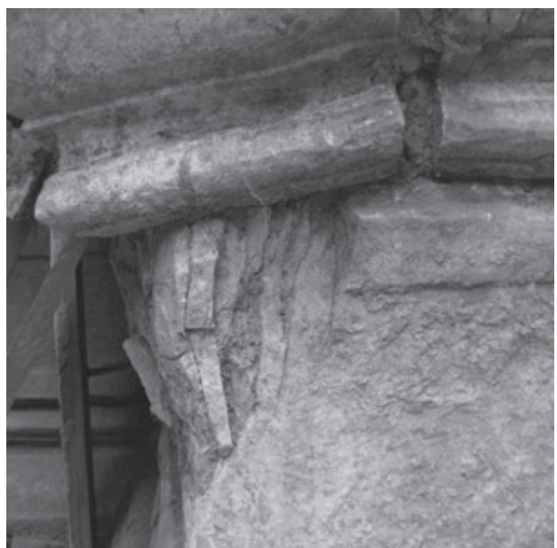
Fig. 39: Damage to a stone panel
